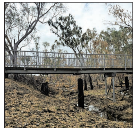
The underside of the bridge at Kanumbra on the rail trail. -S
