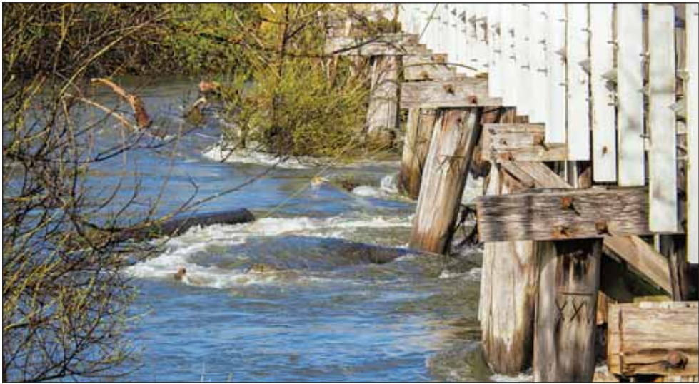
The debris built up beneath Breakaway Bridge on Wednesday, September 28, 2022, immediately prior to the October 2022 flood event. -AR
